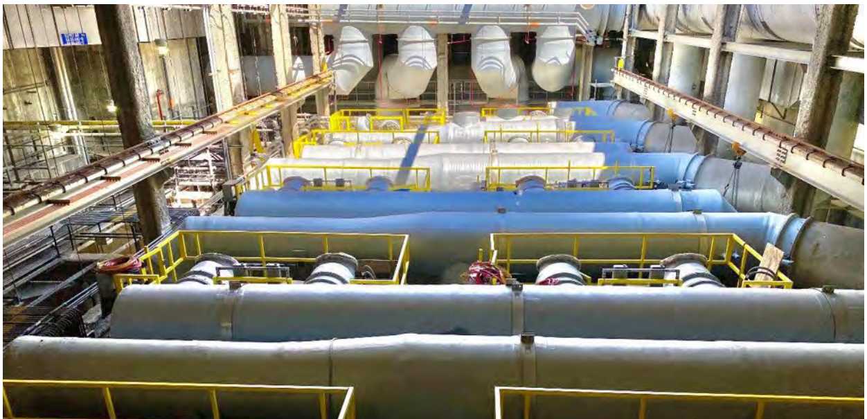
Odor Control Room Showing Platforms and Ductwork above Carbon Adsorbers
