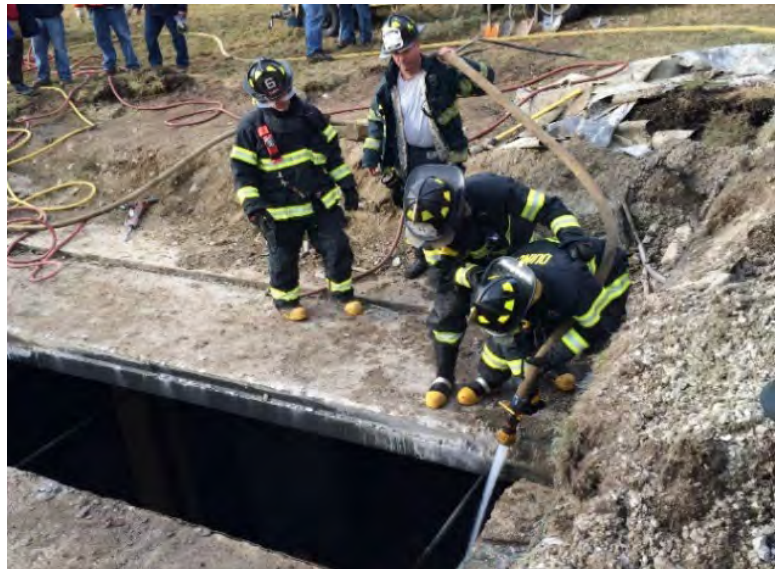
Removal of Subsurface Roof Required to Access Odor Control Room during January 2016 Fire
